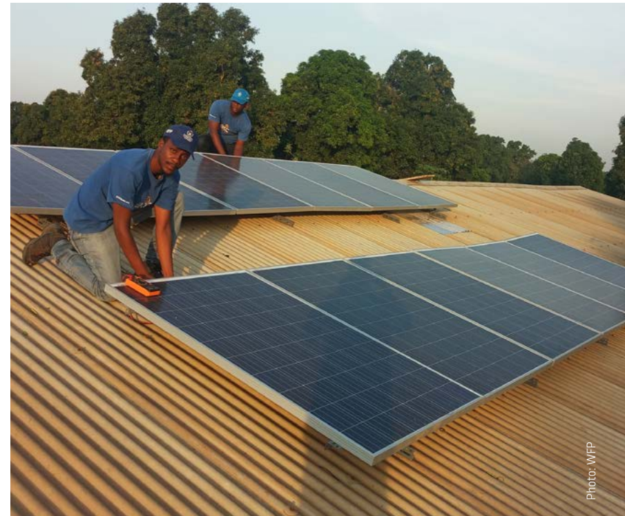
The ETC deployed to Batangafo, CAR to install a solar panel system to supply a reliable power source for emergency.lu satellite equipment, which provides connectivity services.
